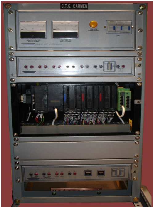
DIGITAL MASTER CONTROL AND RECTIFIER BRIDGE . BRUSHLESS TYPE
