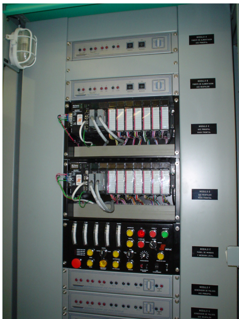
Electronic master controller for 350 MW units. Petacalco power plant
